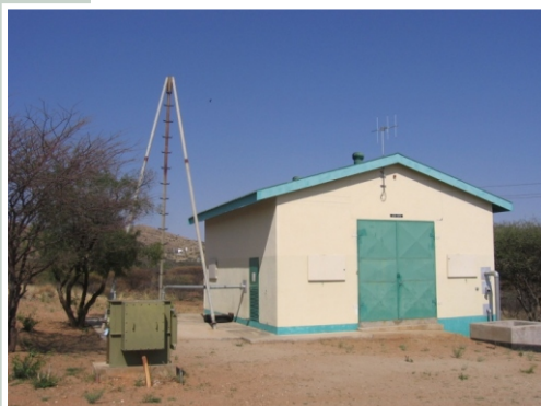
One of Windhoek's injection boreholes (below the tripod) and the water treatment building where further treatment is given through Granular Activated Carbon and chlorination
