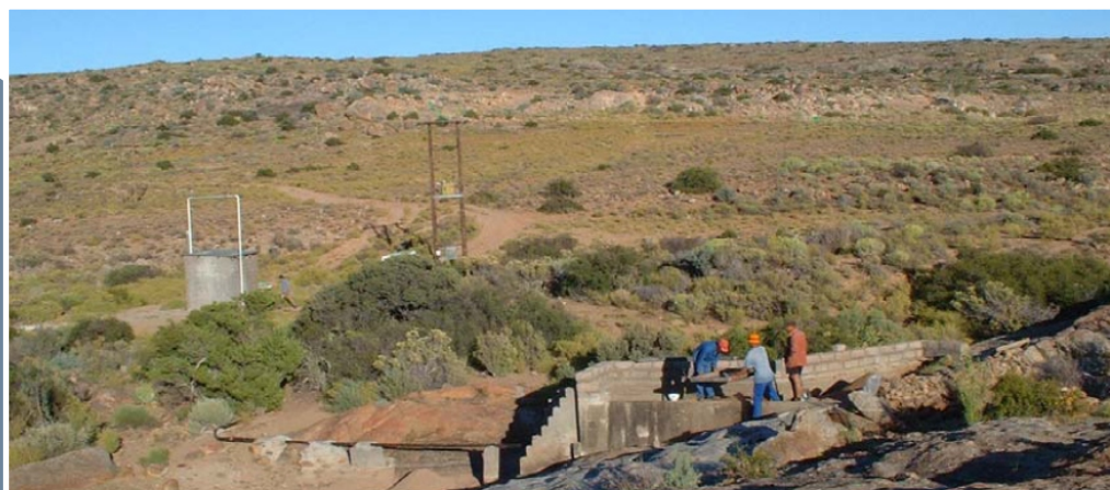
Sand filter with injection and abstraction borehole (pump house) in the background
